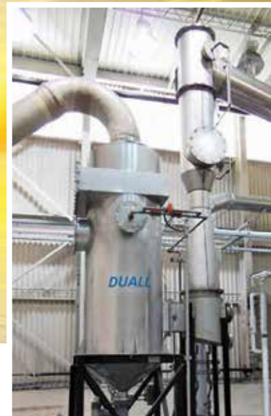
Venturi Scrubber System Treating Emissions from an Industrial Furnace
