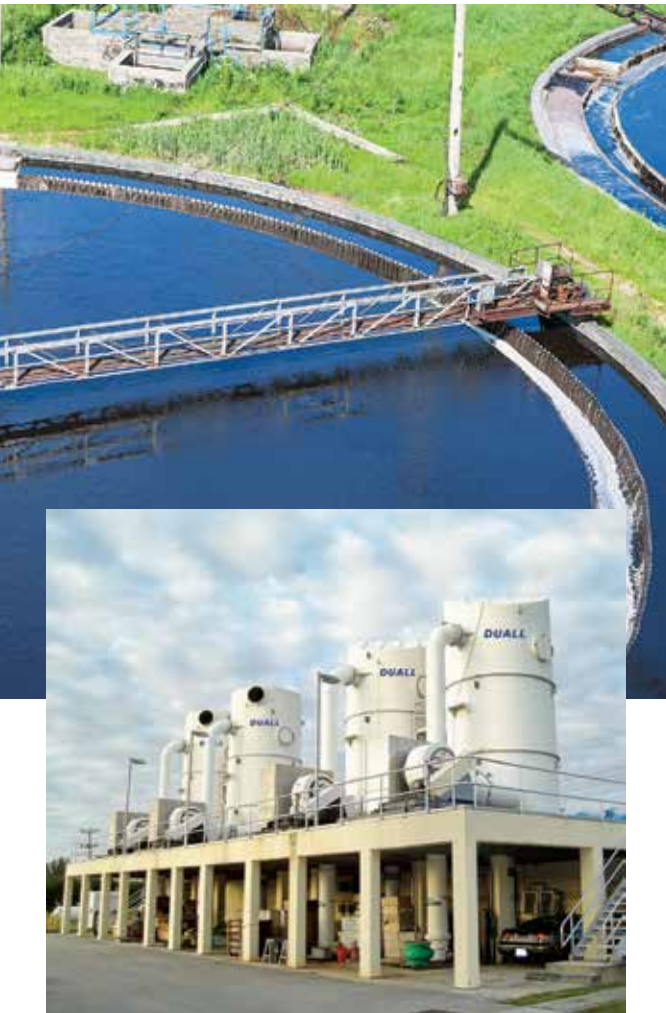
Water Production Plant with Degasifiers
