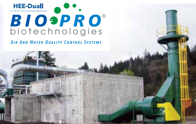
Biofilter Removing Hazardous Air Pollutants (HAPs)
